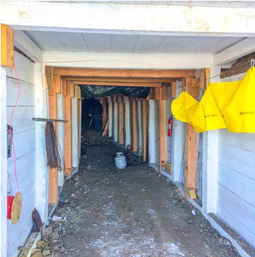
Plate 20: PGM’s refurbishment of the first 50 meters of the historic 700 level in the Empire Mine during 2018
